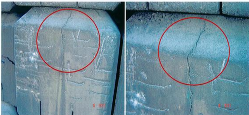
HORIZONTAL & VERTICAL CRACKS. REJECT
